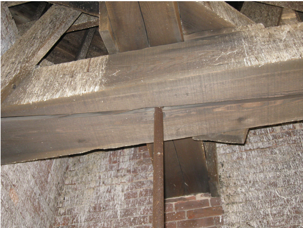
Wood structural support beam with significant cracks the length and depth of both beams. Structural steel tension rods which provide stability and support are loose and not effective. Wood beams are pocketed into brick wall with loose brick and mortar
