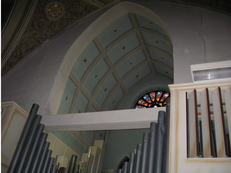
Significant cracks in plaster on both sides and ceiling of choir area. Plaster cracks are representative of the brick steeple located directly behind this wall. These cracks reported by parishioners in 2011 and are what prompted the initial structural assessment of the steeple.
