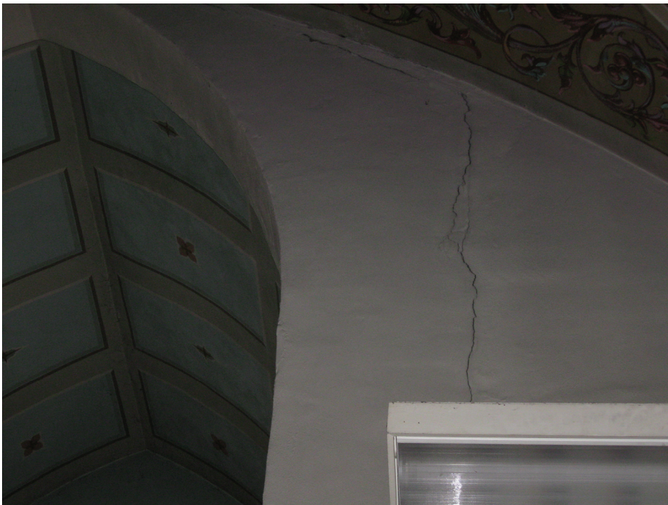
Close up photo of plaster crack in choir loft. It is important to note these cracks appeared suddenly and prompted a structural assessment which identified dangerous conditions. This condition documents movement of the church steeple and is consistent with the structural engineering findings of major cracks in structural wood beams, loose steel tension rods and structural damage to the brick exterior walls. It should also be noted this was a sudden event and not due to lack of maintenance.
