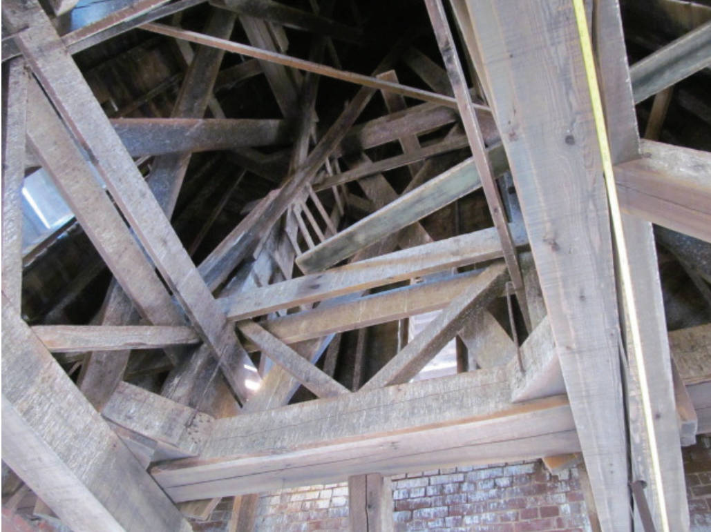
Main wood structural support beam with significant crack through the entire length and depth. Steel tension rods which pass through the wood beam are loose. This condition is not due to the lack of routine maintenance.
